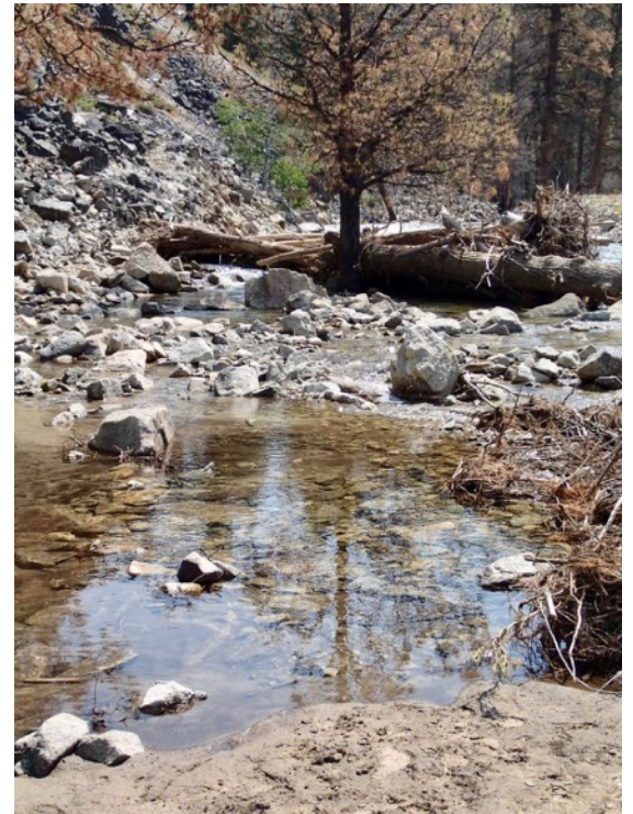
Washout closing Nf-227 east of Baumgartner Hot Springs.
