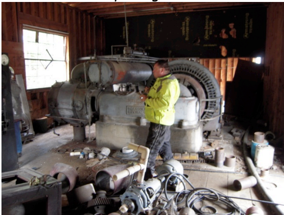
Example of old machinery and parts found in the buildings of the mid mountain area.
