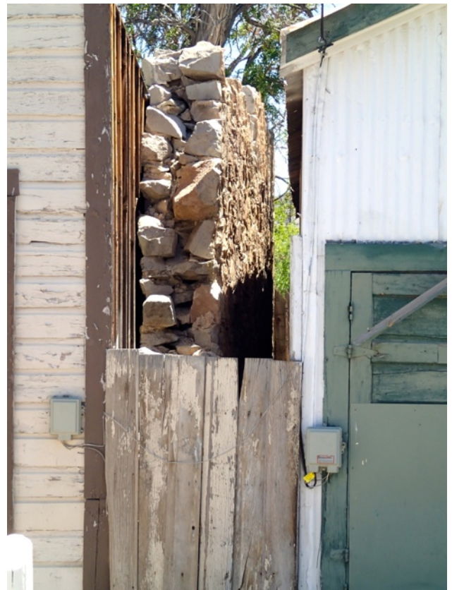
Original rock wall of the Overland Stage Station and Pony Express stop located to the west of the Union Hotel.
